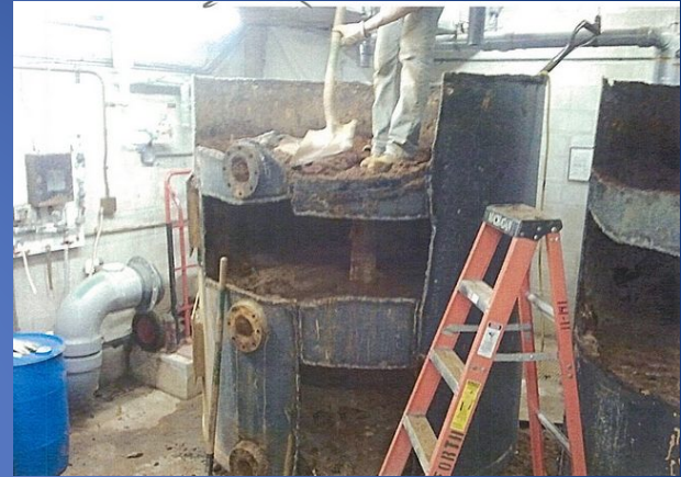
OLD SAND FILTER
